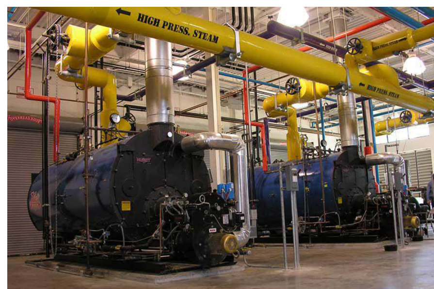
Boiler and pressure plant
